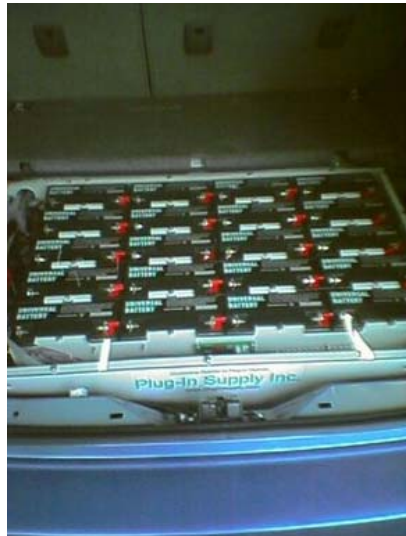
Figure III.6 Lead acid batteries. Source: Plug-in Supply Inc
